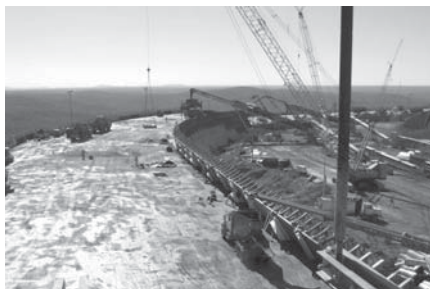
AmerenUE continues to work on rebuilding its Taum Sauk Pumped Storage project after a 2005 incident.
