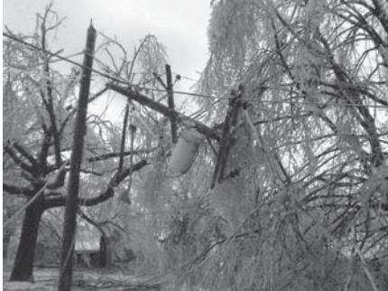
This photo shows some of damage the 2007 ice storm caused to the service territory of The Empire District Electric Company.
