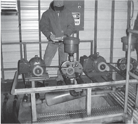
PSC staff member Jerry Scheible inspects a motor and blower assembly on a mechanical sewer treatment plant.
