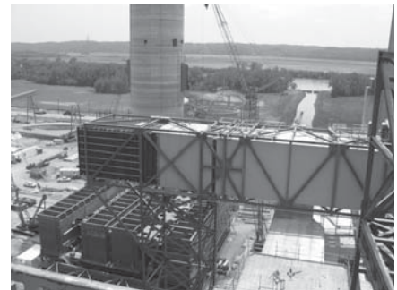
Work continues on the new Iatan 2 power plant near Weston. The plant is being constructed by Kansas City Power & Light Company.
